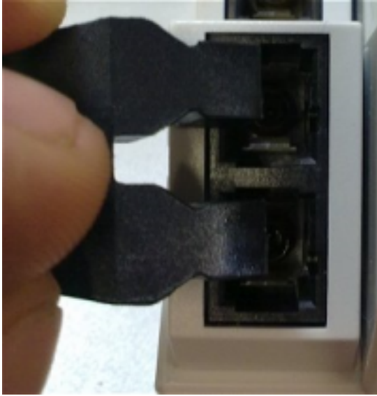
Figure: Blind plugs in unused sockets
